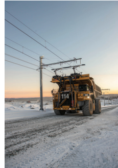
Boliden's project conducted since 2018 in Aitik has seen 700 meters of electric trolley line installed with the conversion of four mining trucks
