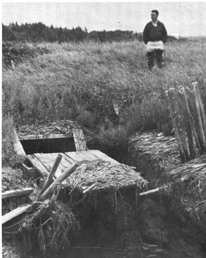
FIGURE 5. A water control structure (aboiteau) on a dike near Kamouraska. The flapgate has become non-functional from accumulation of tidal trash.
